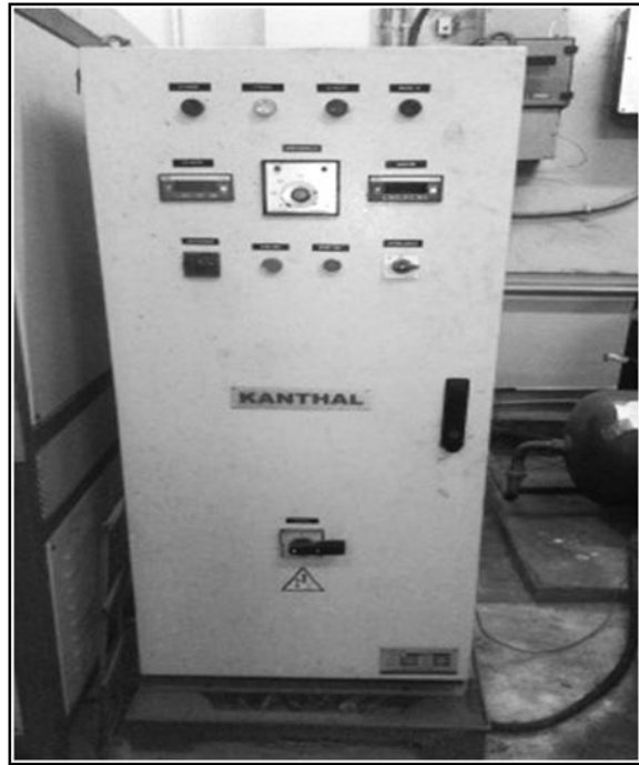
Fig. 3.1.2 Furnace Control Panel
