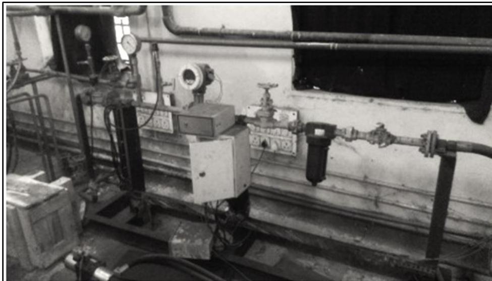
Fig. 3.1.7 Compressed air flow circuit with digital flow meter
