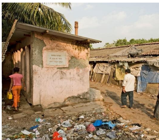
Plate 5.q: Toilet facility of Madhobtala slum, Dhakuria (Along the Railway Line, Unregistered Slum)
